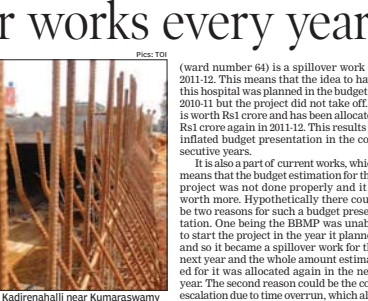
CARRY OVER: The construction of a grade separator at Kadirenahalli near Kumaraswamy Layout appears to be a perennial project as it has been pending for four years now
